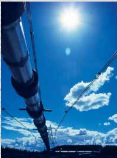
Oil & Gas pipe
